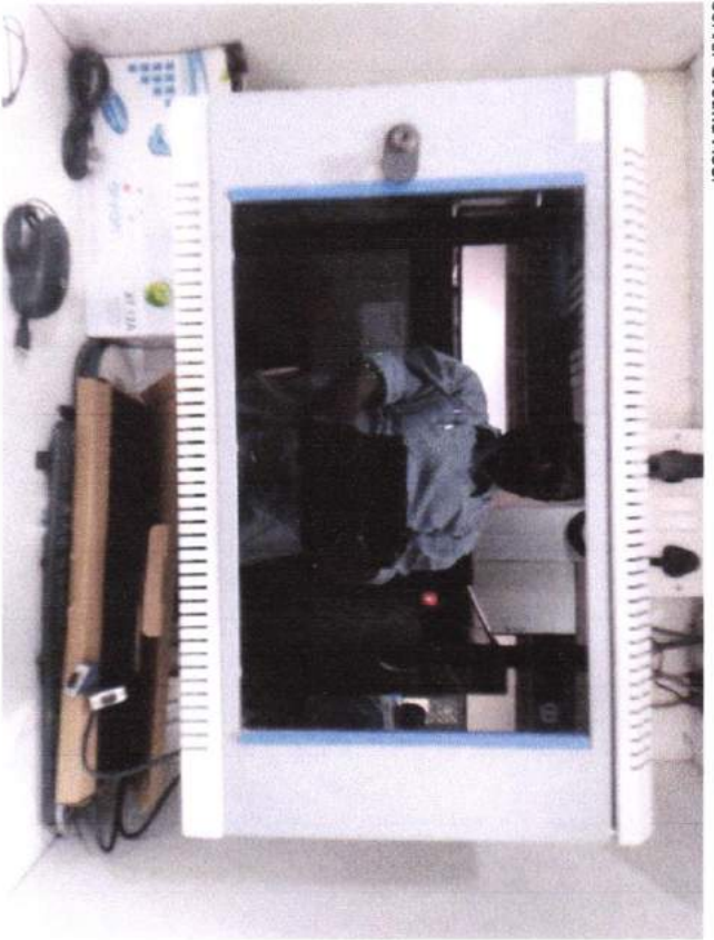
Server Ground Floor
