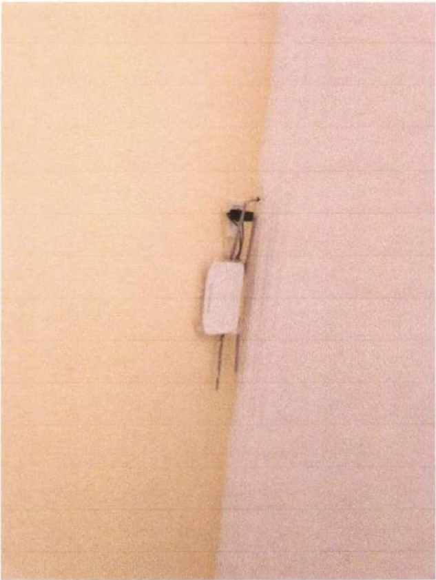
Wifi Router 4th Floor 2
