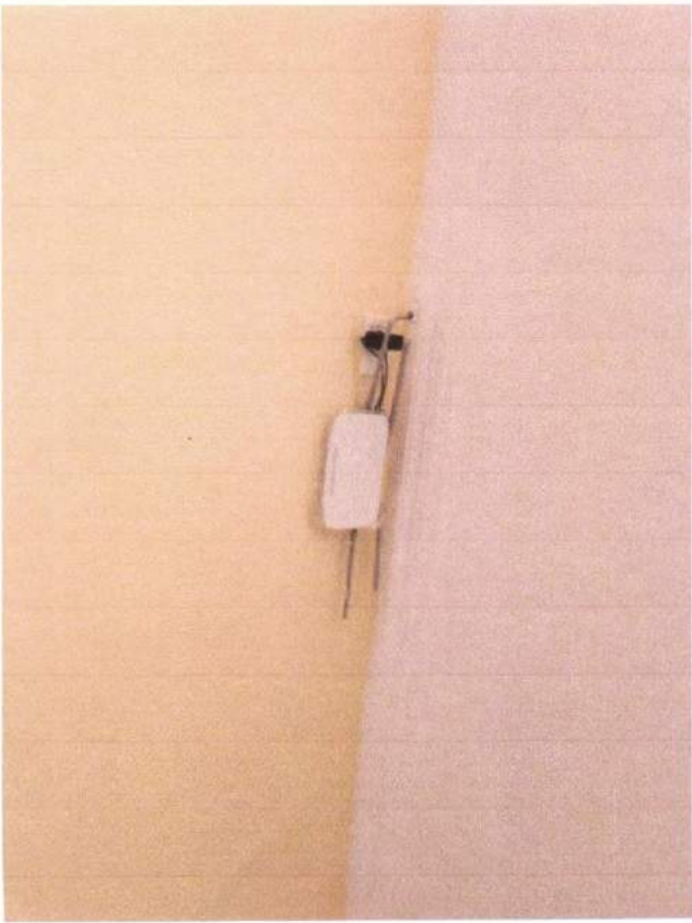
Wifi Router 5th Floor 1
